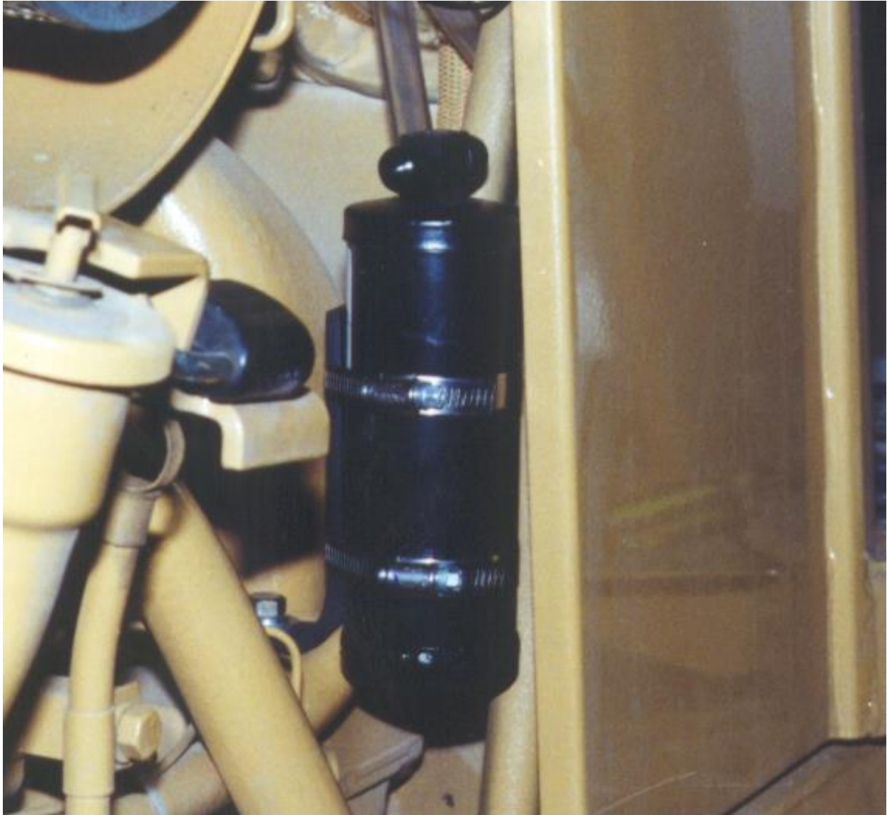
Drier in place.
