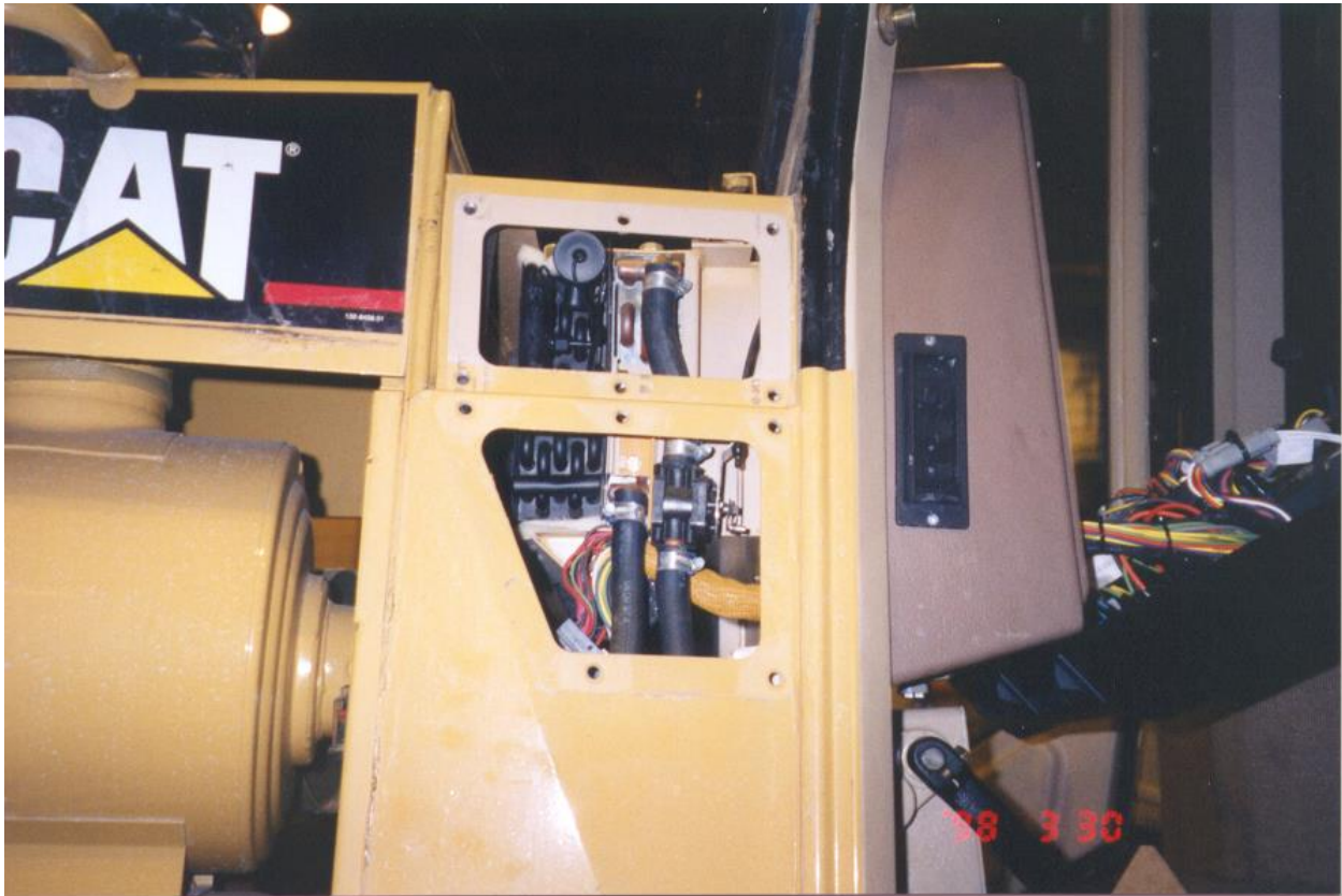
Evaporator in place alongside heater coil.
